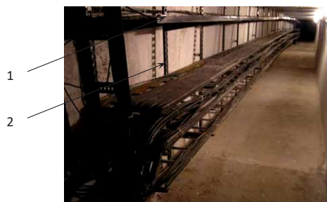
Fig. 1. Cable tunnel with a one-side cable laying: 1 – cable lines, 2 – armature for cable lines laying
